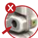
Missing large screw
