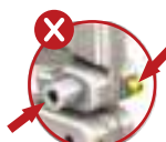
Large or small screws protruding
